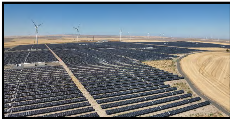
Wheatridge Solar Facility near Lexington
