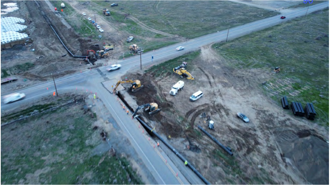
Water lines going in for this airport expansion for new data centers just approved by the county.
