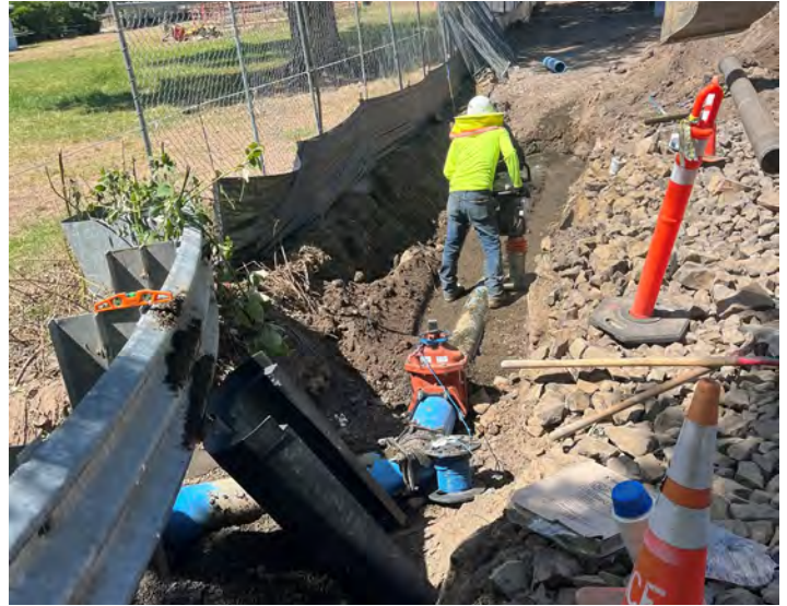
SilverCreek's civil crew installing the main water line prior to making the utility bridge crossing.
