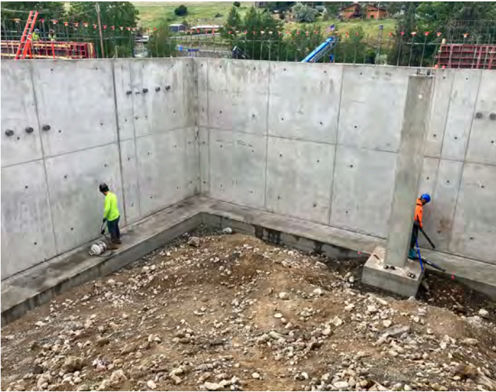
RJ Construction prepping and cleaning the top of footing prior to install of the interior retaining wall waterproofing.
