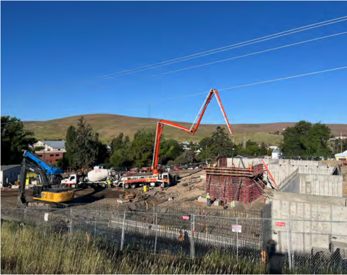
SilverCreek's concrete crew pouring the first lift of the center stair wall on Thursday May 21.
